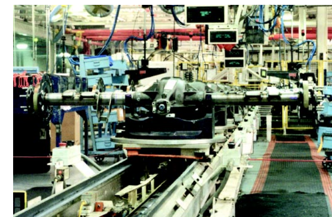
CARTRAC installation at American Axle facility interfaces with both manual and robotic operations.
