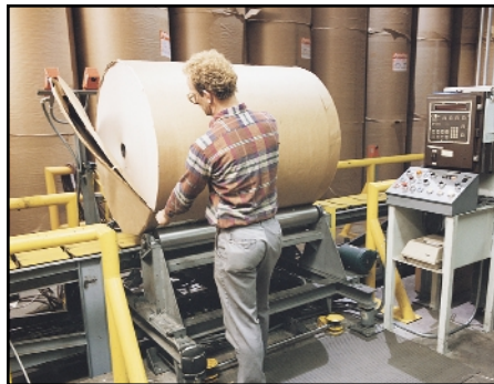
Figure 3: Strip, de-head, and automatic roll weighing devices with controls can be provided prior to or after laydown areas.
