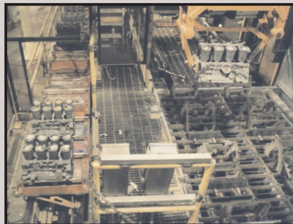
Figure 5: In this core assembly foundry installation Robolite demonstrates that it functions well in a harsh environment.
